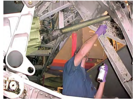
Zip-Chem recommends assessing the condition of every airframe and powerplant for corrosion issues prior to parking it. Zip-Chem image.
